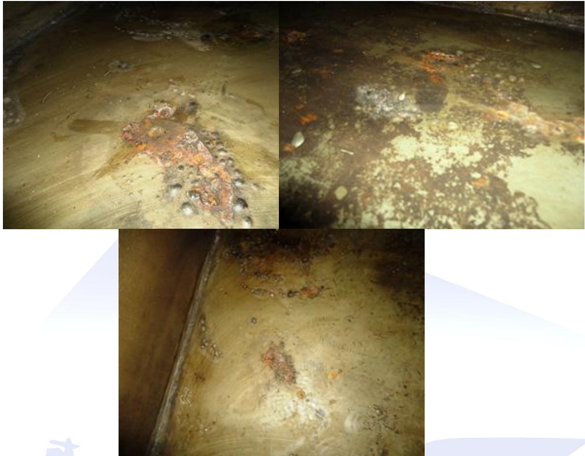
Figure 5 Coating defects and pitting corrosion.
