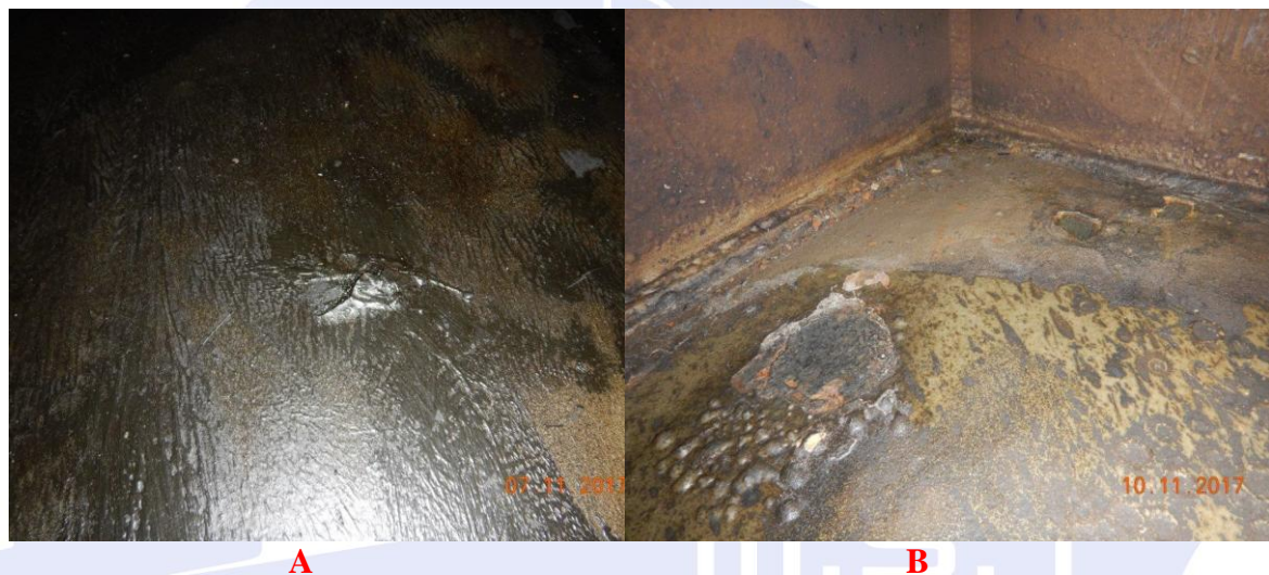
Figure 3 Coating failure due to the presence of the SRB on the bottom plate.
